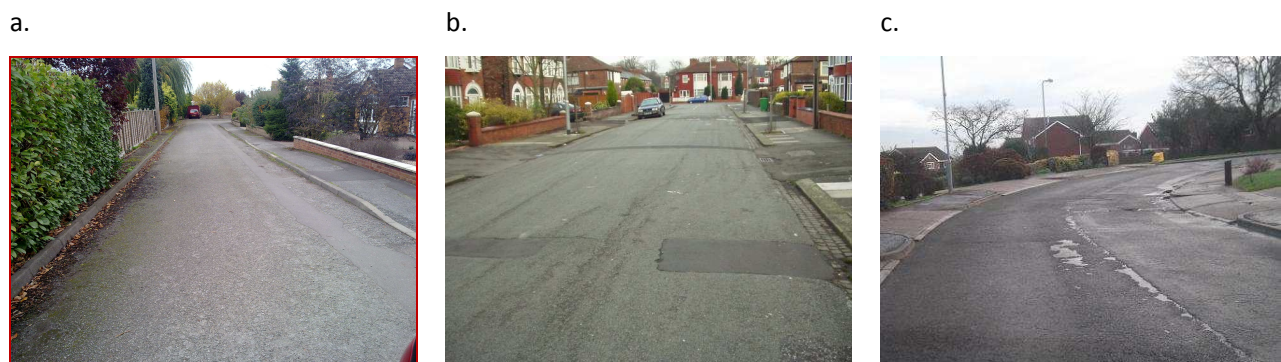
Photo's illustrating a range of amber1 and amber2 condition roads (includes need for surface dressing (a) and Micro Asphalt (b))
