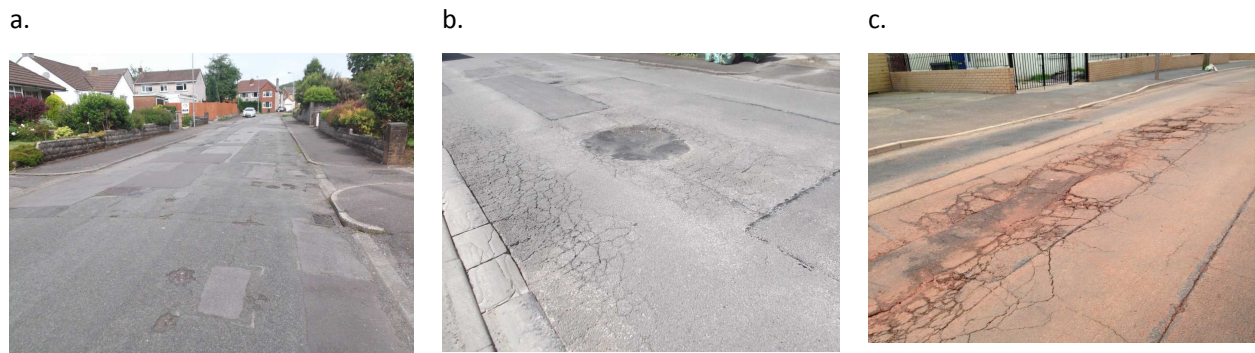
Photos illustrating a range of red condition roads (includes need for resurfacing (a) & reconstruction (b & c))
