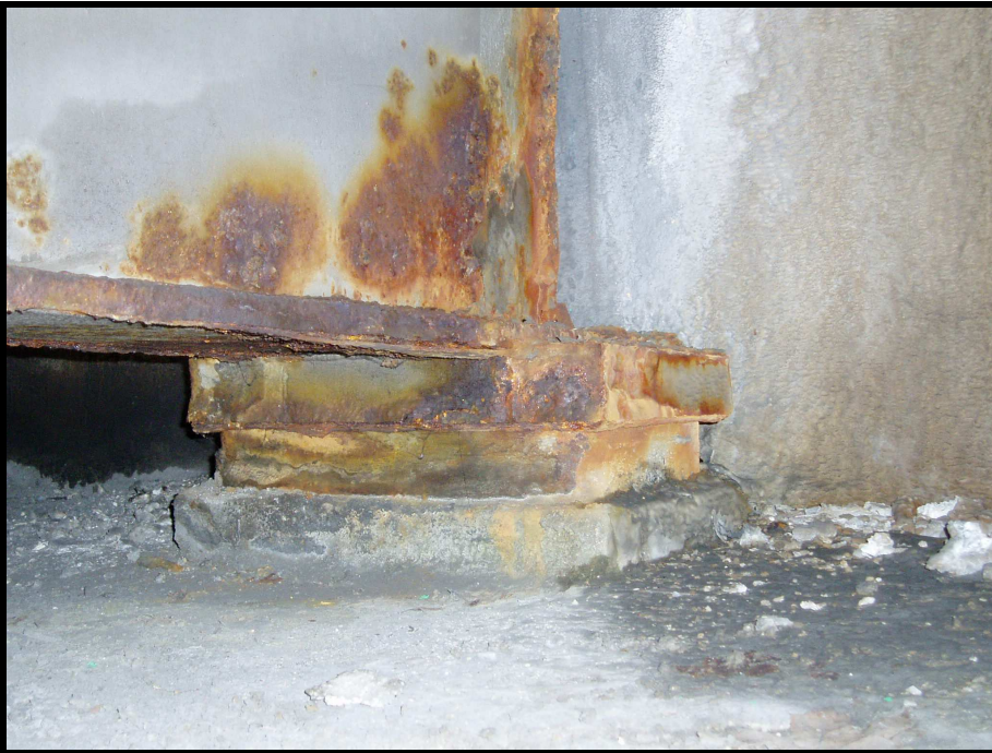
(Corrosion, loss of section and reduction in strength)
